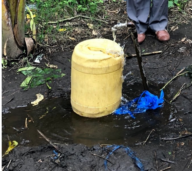
Figure 16: Broken public water tap.
