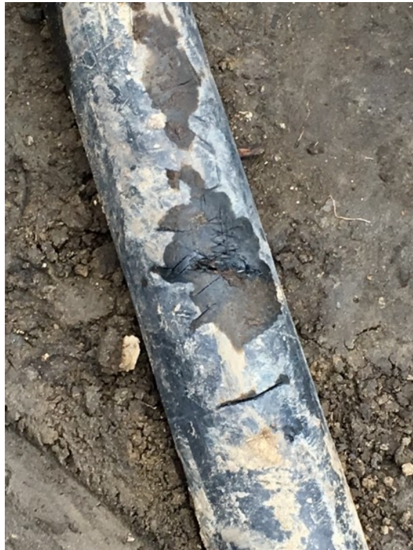
Figure 15: Exposed and damaged water pipe.
