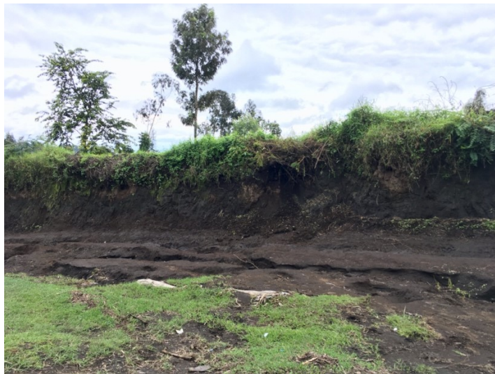
Figure 18: Road erosion in Olkokola. Road to the division box in Engorika.
